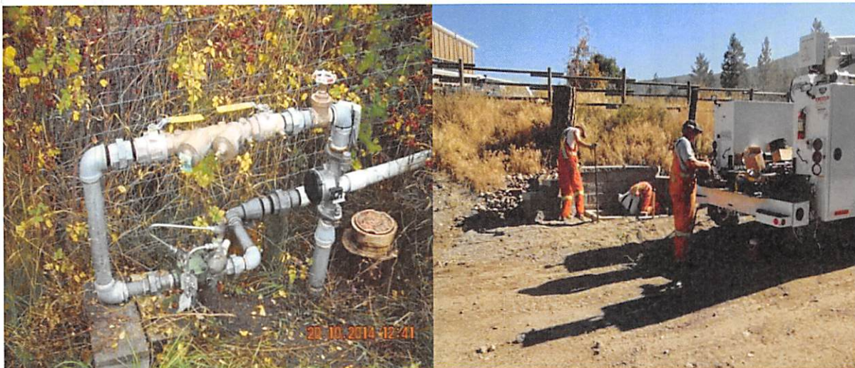
Neptune Meter and Apollo Backflow installed (left) and District installing a Meter and Backflow unit (right)
