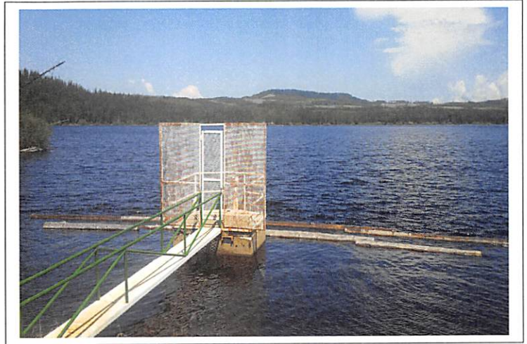
Beaver Lake Dam Intake
