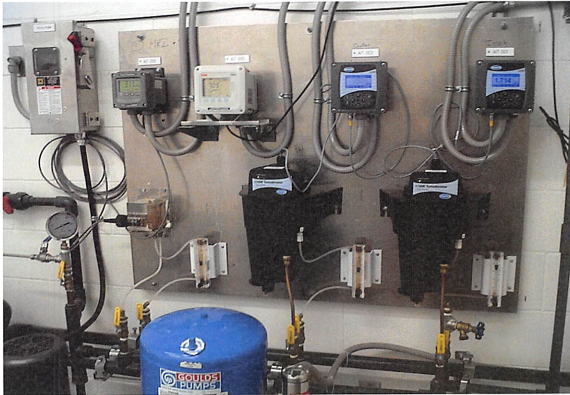
Water chemistry equipment (residual chlorine and turbidity meters) at Eldorado Balancing Reservoir (above).
