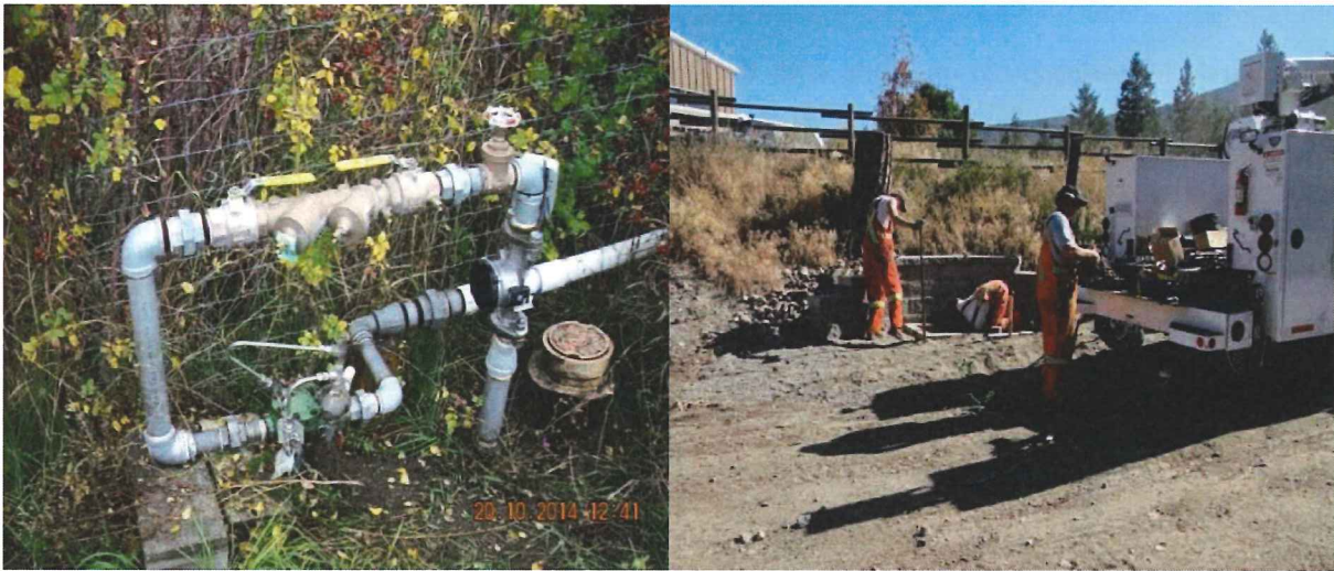
Left: High Volume Ultrasonic Meter and Backflow installed. Right: District installing a Meter and Backflow unit.
