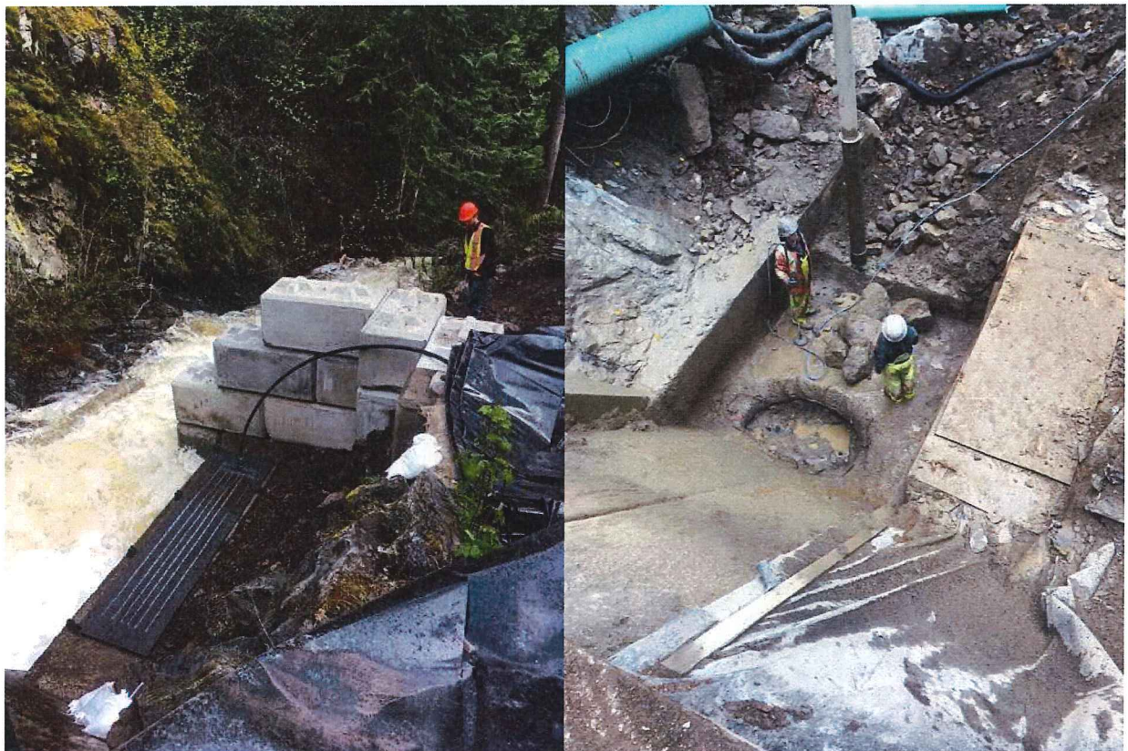
Left: Construction of temporary dam directly below debris filled Oyama Creek intake. Right: Damage to the spillway caused by the extreme flows.
