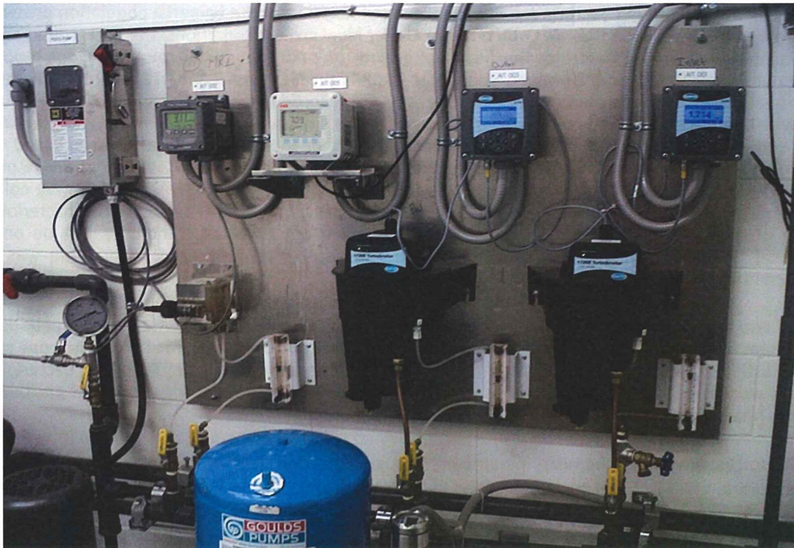
Water chemistry equipment (residual chlorine and turbidity meters) at Eldorado Balancing Reservoir
