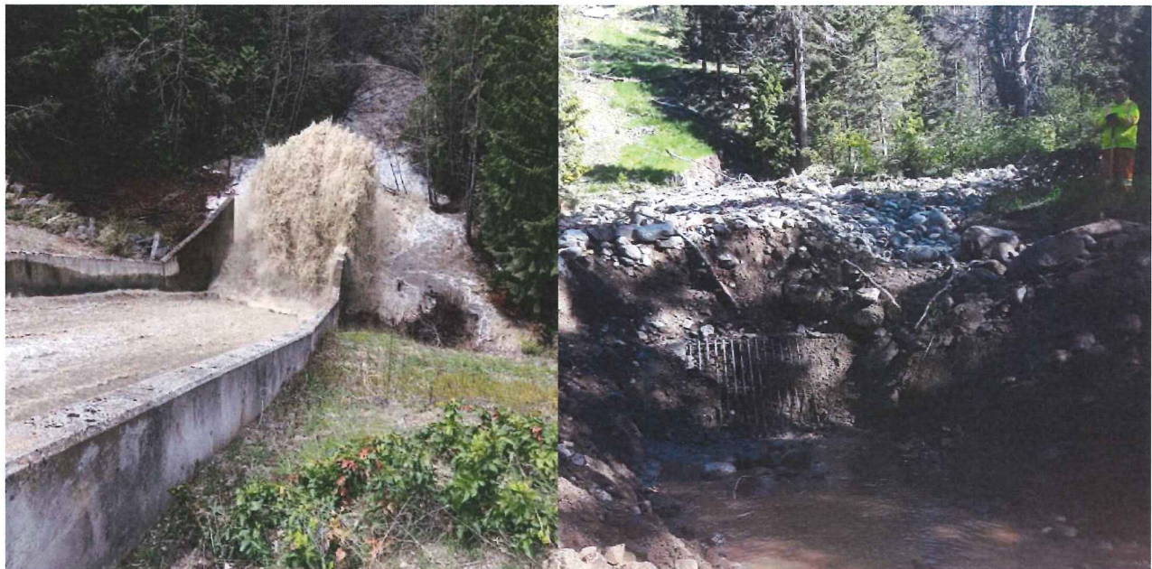
Left: Vernon Creek spillway during high flows. Right: Eldorado overflow outlet structure uncovered but still full of sediment.
