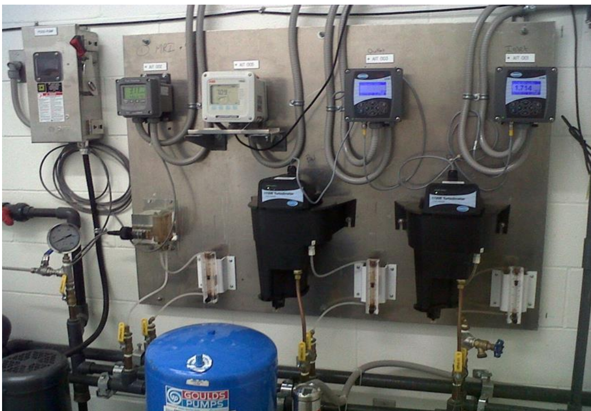
Water chemistry equipment (residual chlorine and turbidity meters) at Eldorado Balancing Reservoir
