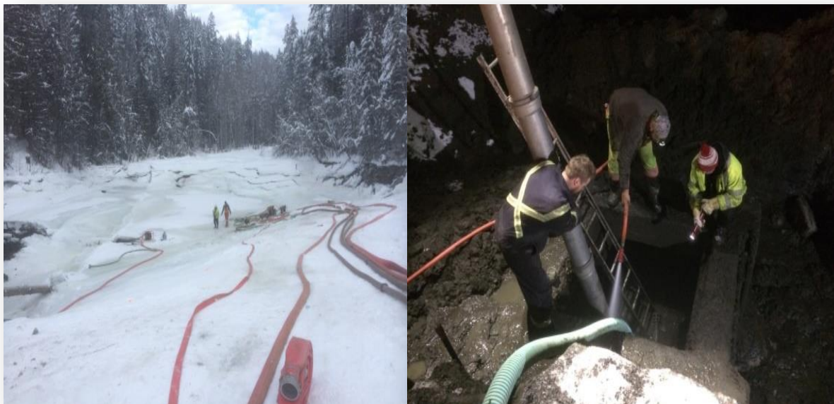
Left: Pumps de-watering the intake pond Right: Hydro-vac excavation of the intake drain box
