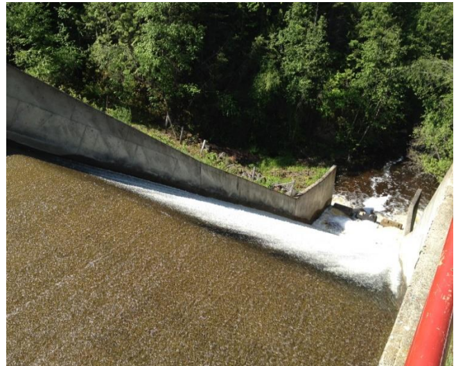
Right: Vernon Creek Intake
