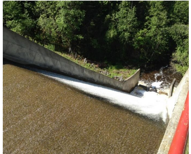
Right: Vernon Creek Intake
