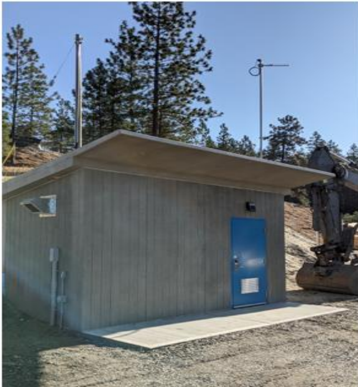
New Hare Road PRV Station
