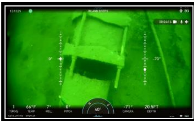
Overhead view showing 4 to 6 inch gap offshore
