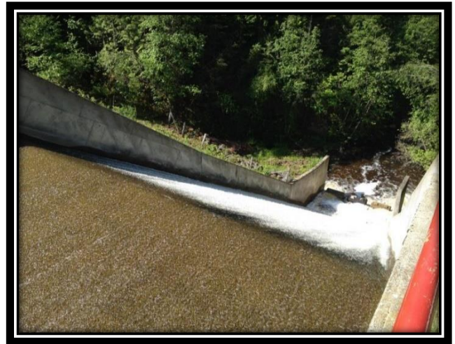
Vernon Creek Intake
