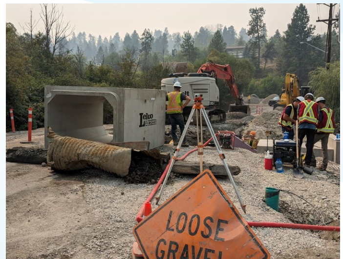
Installation of a new concrete box culvert to replace aged pipe culvert on the west end of Woodsdale Road.
