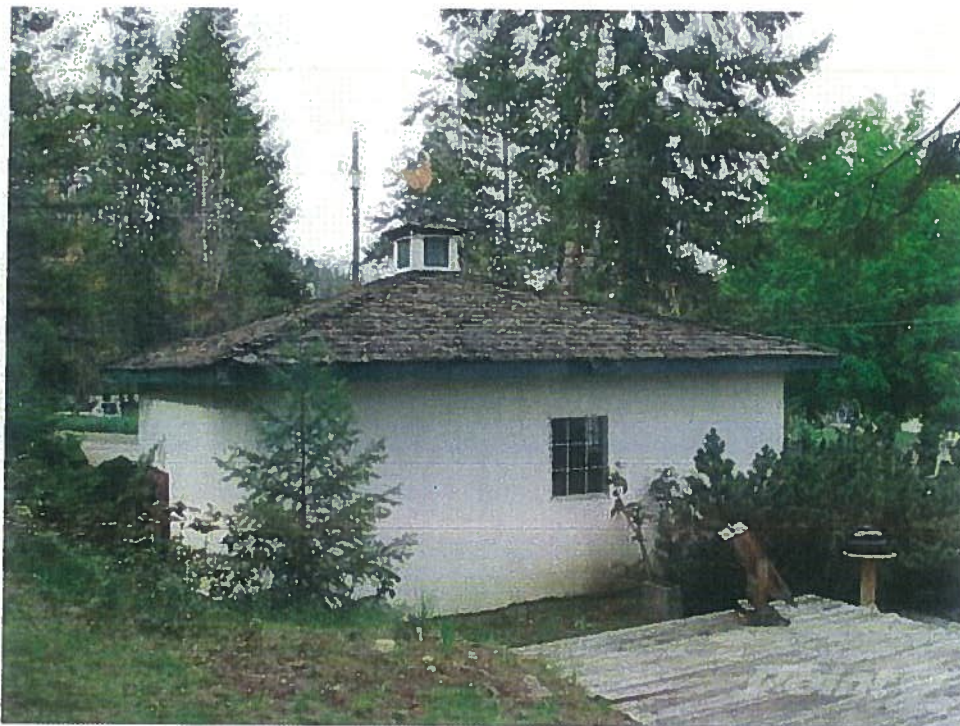
Figure 12. Photograph of an unrated roofing material present on some homes within the wildland urban interface.
