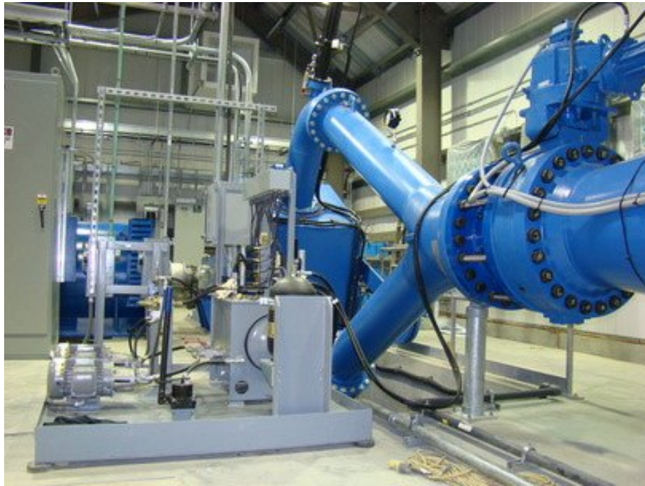
Photo 5 - Incoming Penstock, Turbine Housing and Generator
