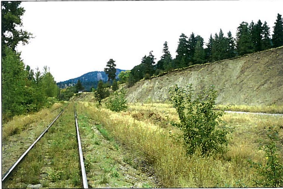
Photo 1: Facing north over northerly end of property. CNR R/W on west property boundary, headwall of former ballast pit on east. The northerly end of the over-steepened escarpment has little vegetation cover and portions over-hang at the top.
