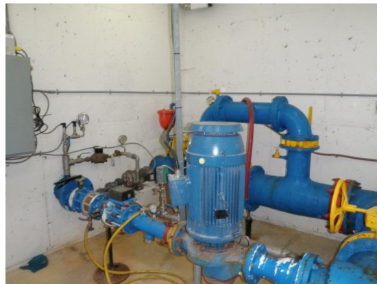
Site 2 Booster Station
