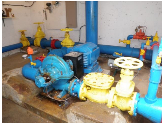
Site 1 Booster Station
