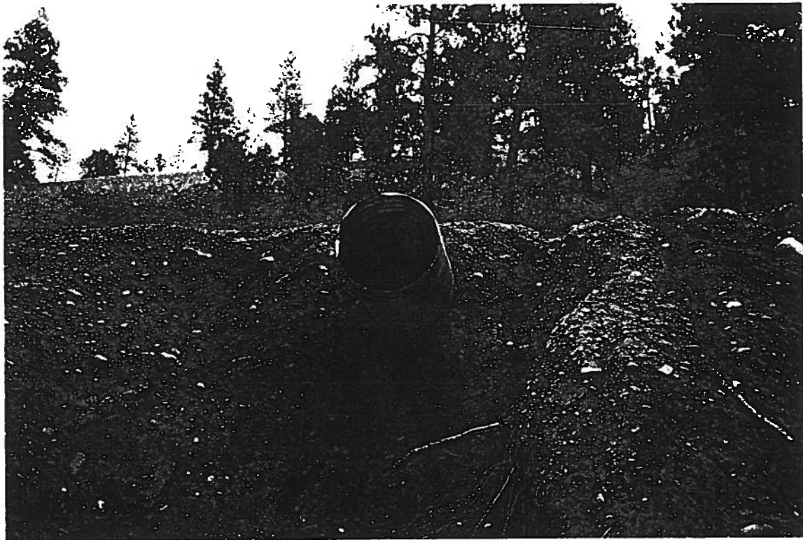
12-10 OK Centre Road West @ Fourteenth Street (Outlet)
