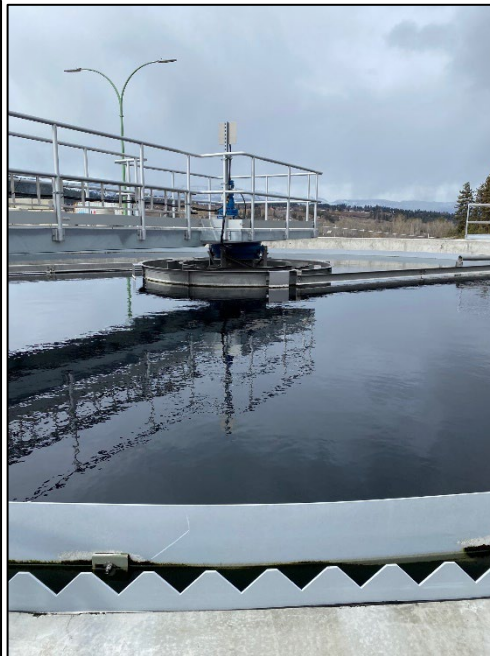
Figure 4: New Secondary Clarifier
