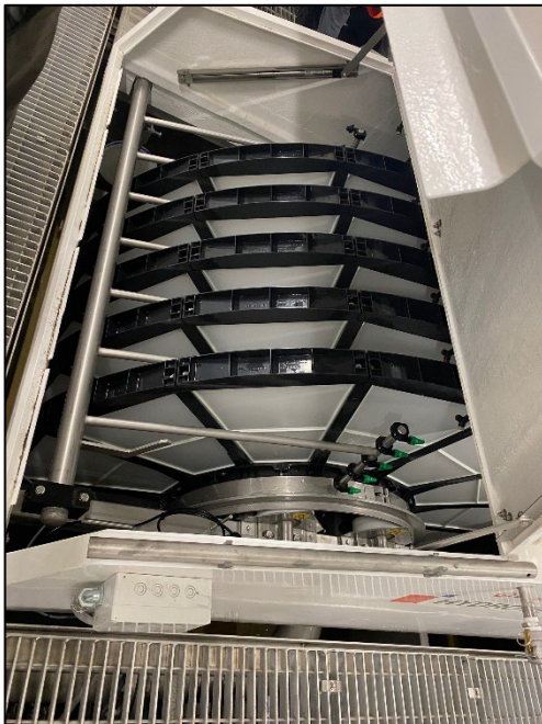
Figure 3: Effluent Disc Filters
