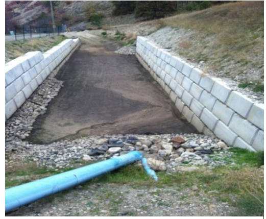
Figure 1: Effluent RI Basin 1
